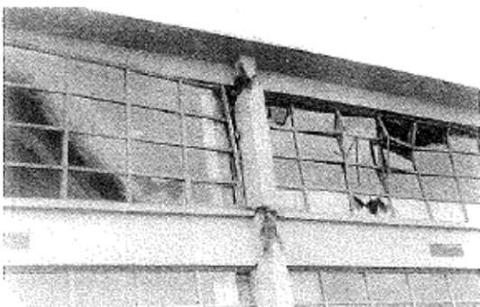
Condition 3: Obvious severe damage to primary structural members, severe racking of wall. Other Severe damage or distress noted.
